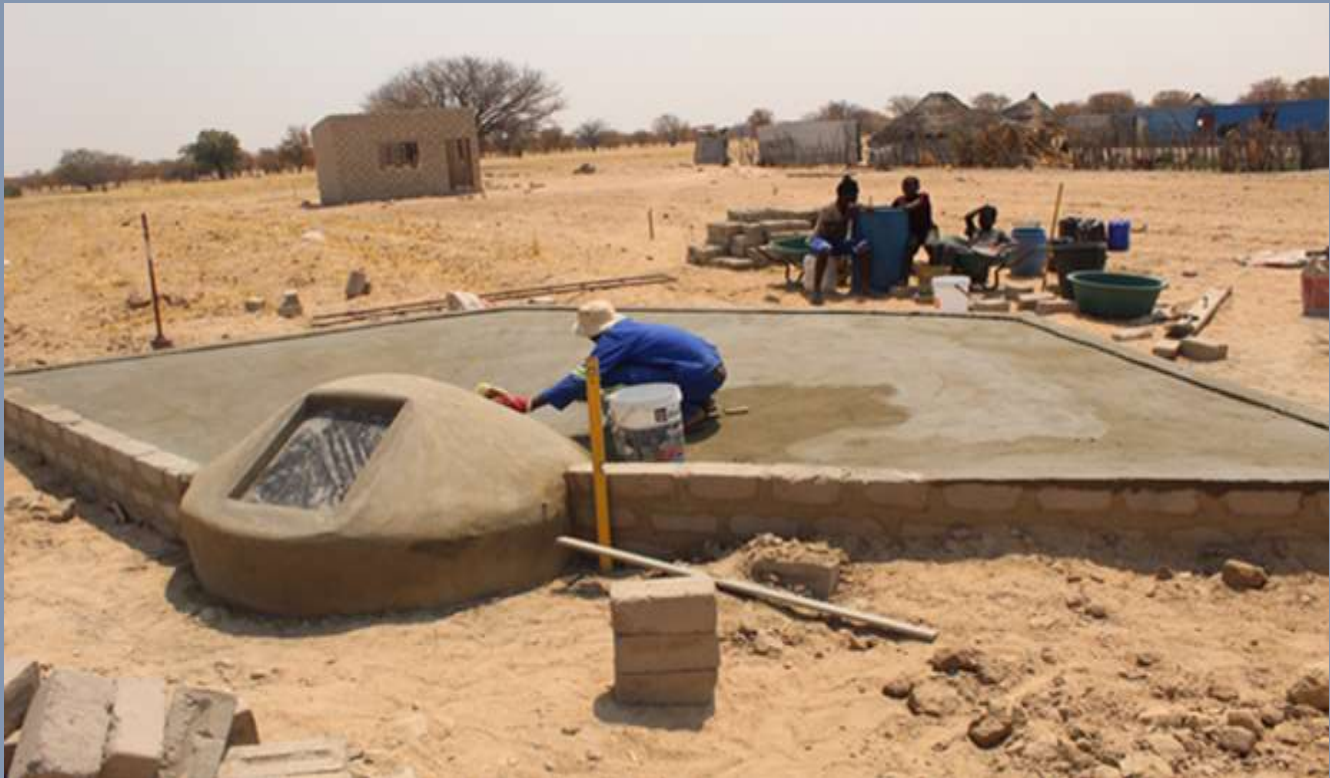
Underground rainwater harvesting system establish in two villages as a demonstration and exemplar to the communities and the local stakeholders
